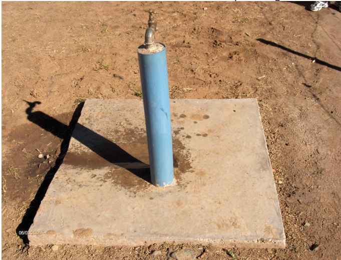
Every yard has a standpipe inside with clean (purified)water.
